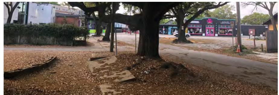
Broken sidewalks creating barriers on Windsor Street in the Cherryhurst area
